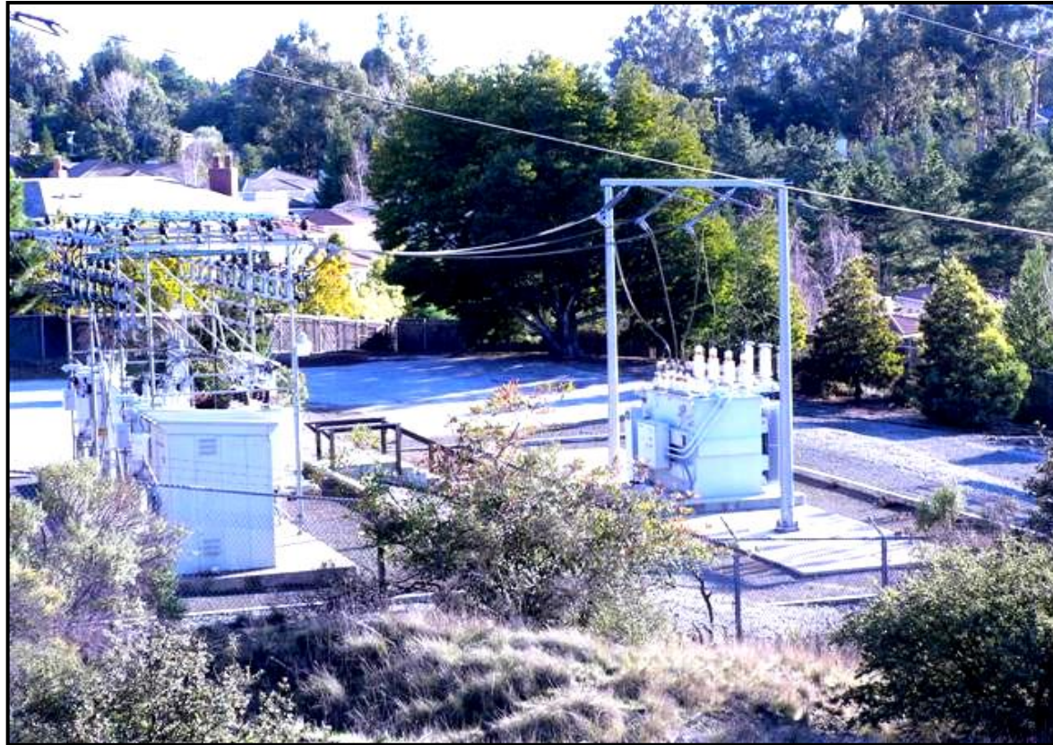
PG&E Emerald Lake Substation
