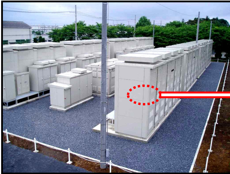
NAS Battery 8MW / 57.6MWh
